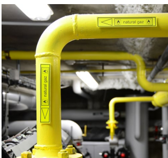
Pipes and valves identification
